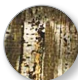
Cracks due to heat
